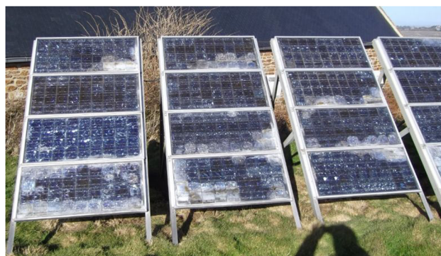
FIGURE 1 Salt deposit on solar panels in coastal climate (photo: Daniel Lincot). [Color figure can be viewed at wileyonlinelibrary.com ]
