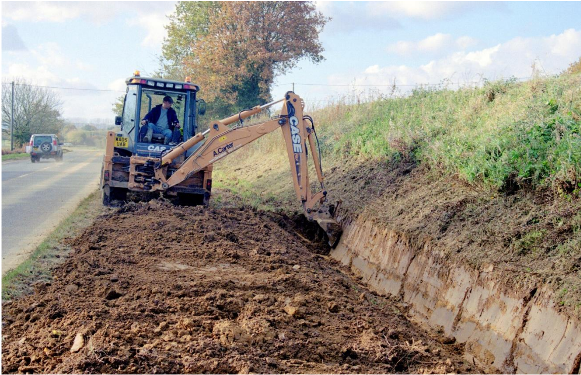
Figure 11. Ditch being dug to protect A272 road from muddy flooding, 01/11/2008, Slade Lane, Rogate, West Sussex
